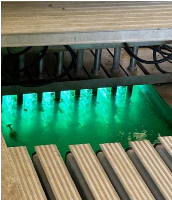
Figure 9. UV light in effluent channel
