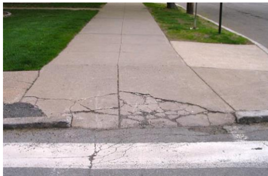
Figure 5. ADA ramp with poor surface condition.
