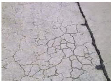
Crack 2 or moderate:
