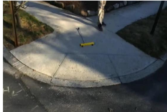
Figure 4. ADA ramp with DWS missing.
