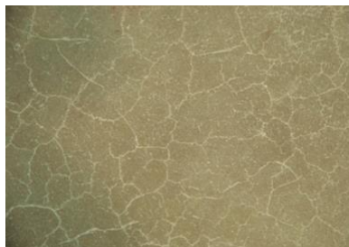
Crack 1 or minor:
