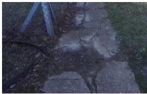
Sample failed sidewalk (0-10)
