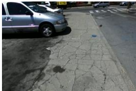
Sample very poor sidewalk (25-40)
