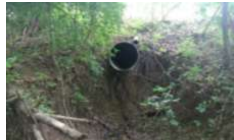
Figure B.1. The above outfalls are examples of different types of outfalls that must be identified on MS4 maps and included in the permittee’s screening program. Areas with highly developed land uses (e.g., commercial business complexes, aging infrastructure) have a greater potential to pollute and must be prioritized. Structural stability and erosion concerns must also be identified as part of an effective IDDE program.
